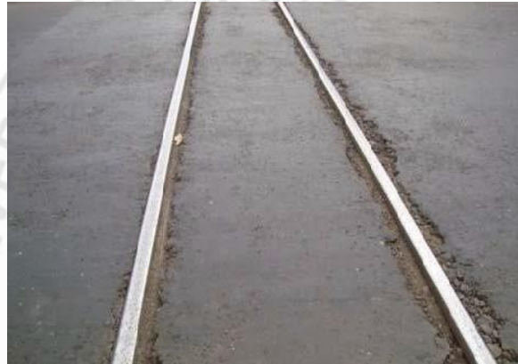
Gambar 2.15 Rusak Perpotongan Rel ( Railroad Crossing ) Sumber: Fitri (2022)
