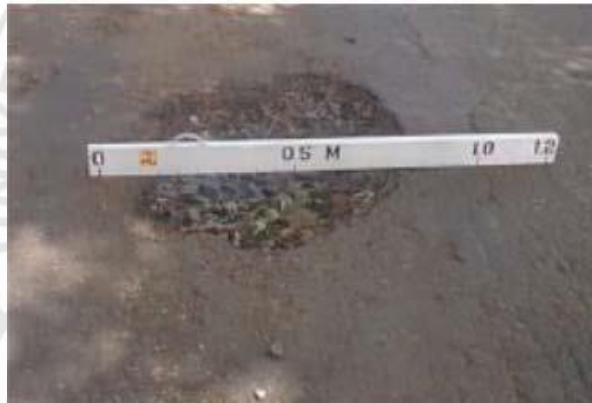
Gambar 2.14 Lubang ( Potholes ) Sumber: Zean (2024)
