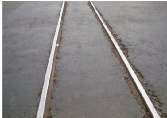
Gambar 2.15 Rusak Perpotongan Rel ( Railroad Crossing )
