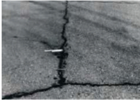
Gambar 2.9 Retak Sambung ( Joint Reflection Cracking )
