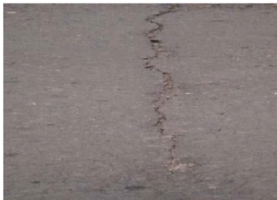
Gambar 2.10 Pinggiran Jalan Turun Vertikal ( Lane/Shoulder Drop Off )
