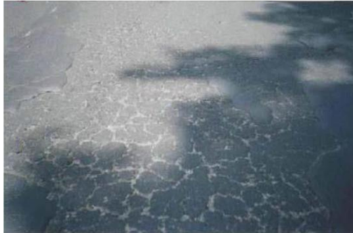
Gambar 2. 19 Pelapukan dan Pelepasan Butir (Sumber : Pavement Management For Airports Roads And Parking Lots , 1994)
